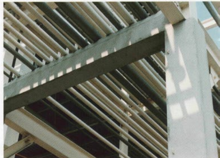
Towelled over lath and cornerbead provides a clean, finished appearance to pipe rack columns.
