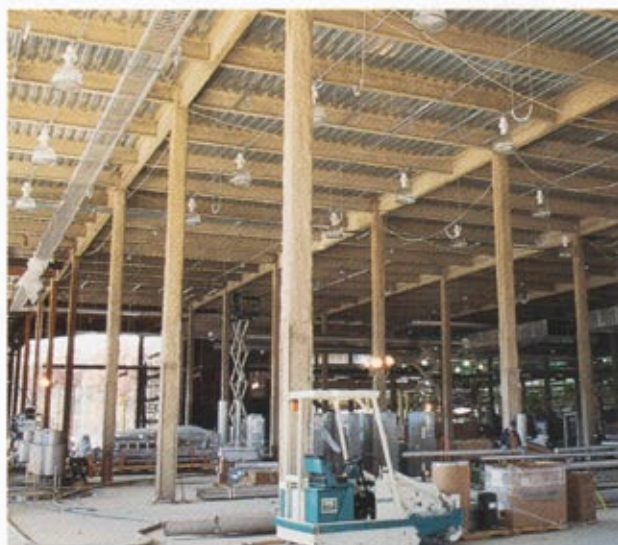
Application of Monokote Type Z-146 during construction of the new Malden Mills manufacturing facility.
