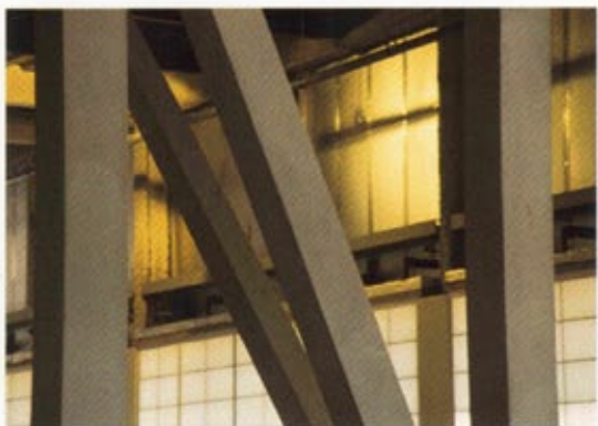
Monokote Type Z-146 trowelled smooth and finished with an epoxy paint provides a washable, dust free surface for a computer chip assembly plant.
