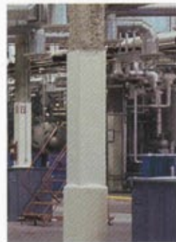
Lower portions of the column have been boxed and trowelled smooth. Upper columns feature a natural, contour sprayed finish.
